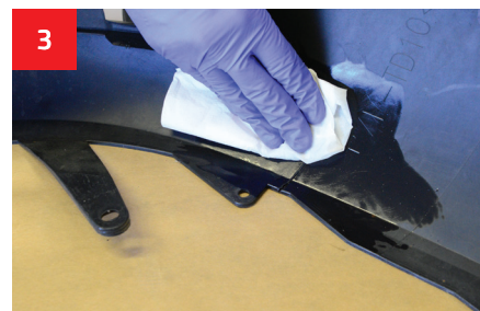
3 Clean and degrease the repair with WK900 on both sides of damage.
