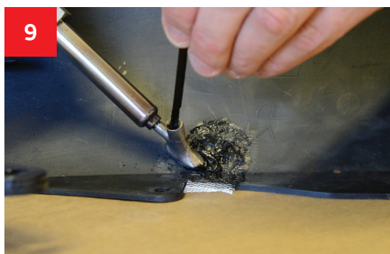
The binding material is set into the damaged area on the inner side of the damage.
