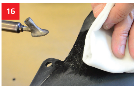
In the case of too rapid melting of the binding material cool down the repaired place with a cloth soaked with cold water.
